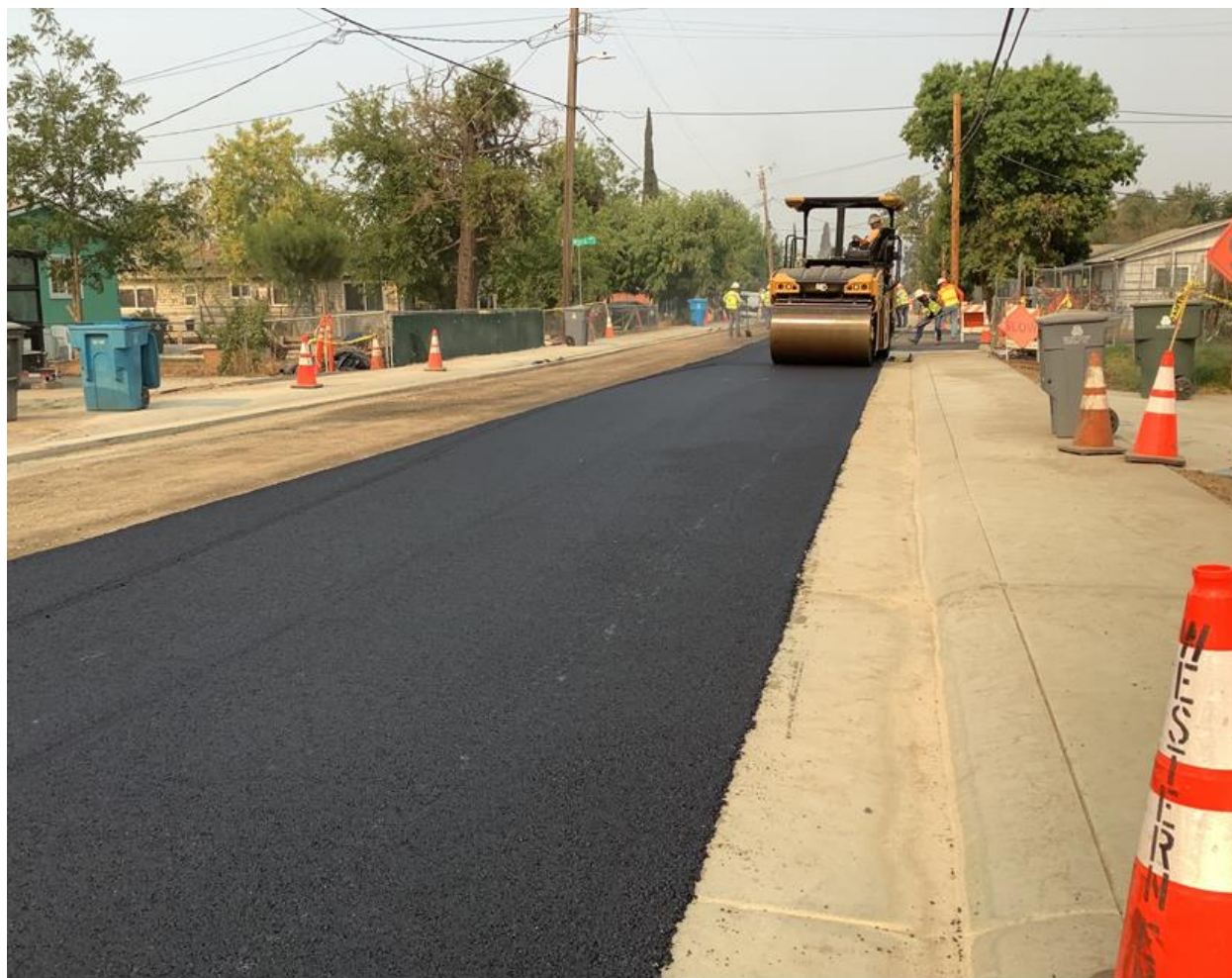
Figure 2-1 Paving After Placement of Curbs, Gutters, Sidewalks, and Storm Drains in mid-2021
